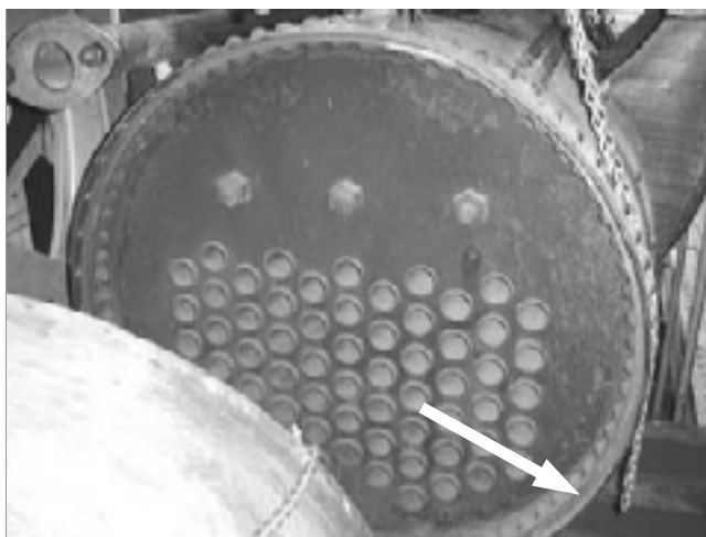
Arrow shows disputed circumferential 'seam' weld position
